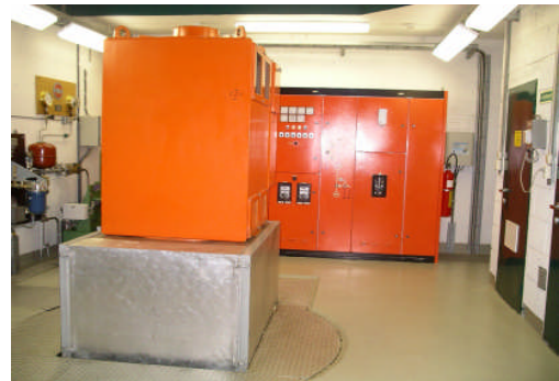
Generator, Sagfossen, Siljan
